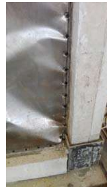
Fig. 9. No rupture of the web plate and no separation from the connecting plate
