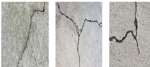
Fig. 3. Some examples of cracked concrete image [28]
