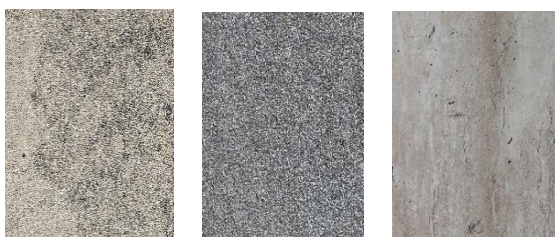
Fig. 4. Some examples of uncracked concrete image [28]
