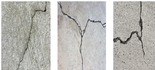
Fig. 3. Some examples of cracked concrete image [28]
