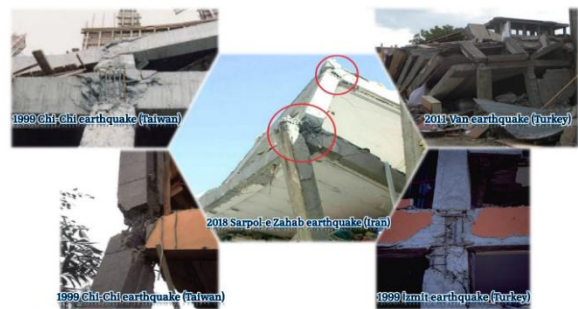
Fig. 1. Damaged RC beam-column connections in earthquake
