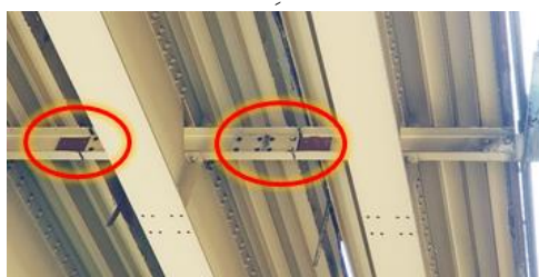
Fig. 3. Removed lateral connections between girders
