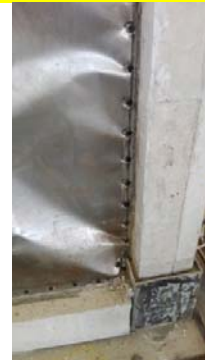
Fig. 9. No rupture of the web plate and no separation from the connecting plate
