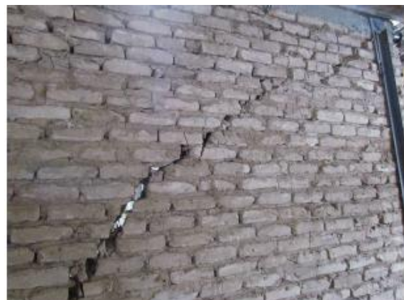
b) Crack opening - back view
