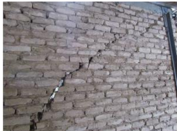
b) Crack opening - back view
