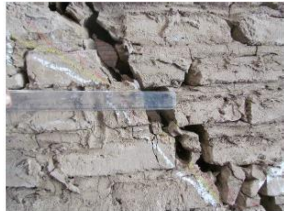
a) Crack opening - front view
