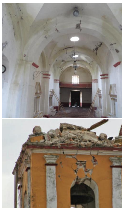
Fig. 22. The distribution pattern of cracks in the field observation of masonry arches after earthquake [۱۵]
