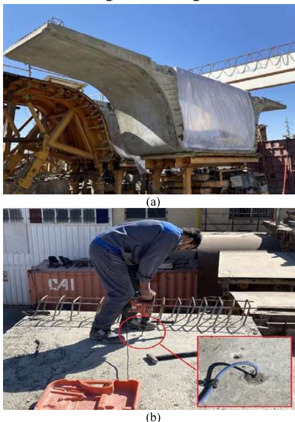
Fig. 5. The experimental concrete-box girder segment: (a) sealed with isolation plastics, (b) drilling and installing thermocouples
