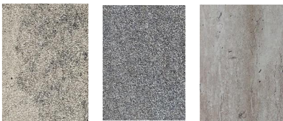
Fig. 4. Some examples of uncracked concrete image [28]
