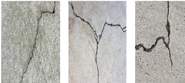
Fig. 3. Some examples of cracked concrete image [28]
