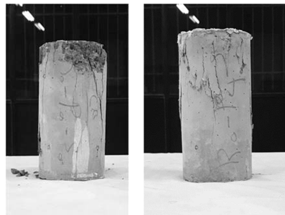
Fig. 7. Scheme of cracking of compressive specimens
