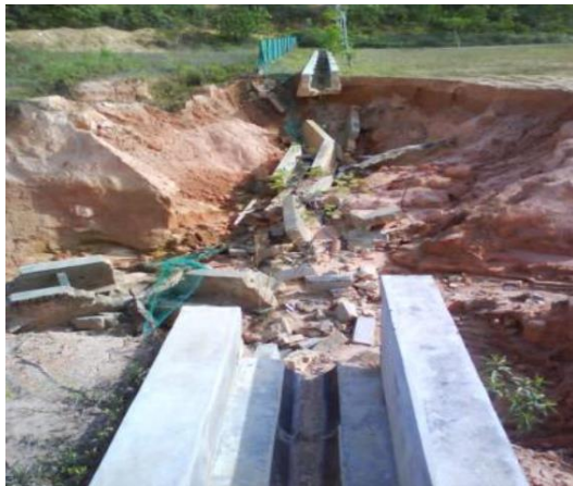
Fig. 1. Water channel failure due to increased soil moisture in collapsible soil [7]
