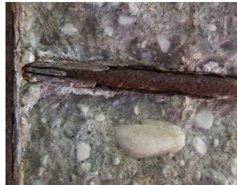
Fig. 1 Uniform corrosion in reinforcement (Bandar-e Mahshahr.)
