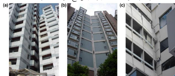
Fig. 1. Pounding damages between adjacent structures, (a) 1999 taiwan Earthquake (b) 2008 Wenchuan Earthquake (c) 2011 christchurch Earthquake [3]
