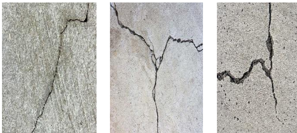
Fig. 3. Some examples of cracked concrete image [28]
