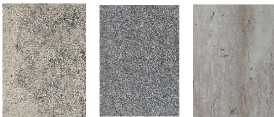
Fig. 4. Some examples of uncracked concrete image [28]
