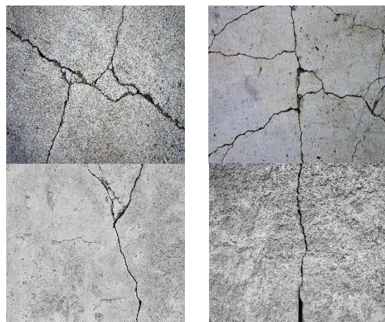
Fig. 10. Sample of cracked images uncracked by incorrect prediction [28]
