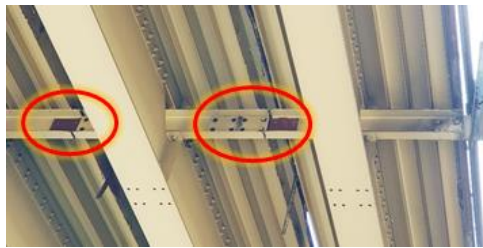
Fig. 3. Removed lateral connections between girders
